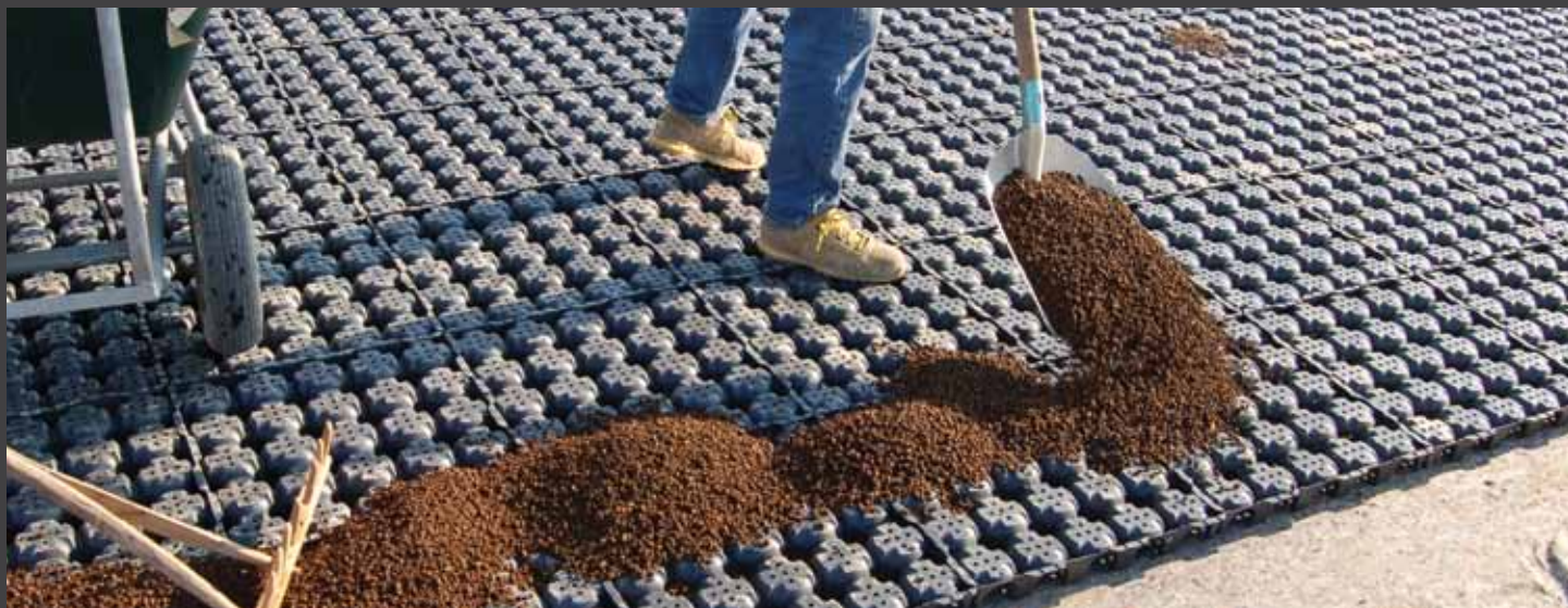
fig. 2) Posa di DRAINROOF e stesura del lapillo vulcanico. Installation of DRAINROOF and laying of the layer of volcanic lapillo.
